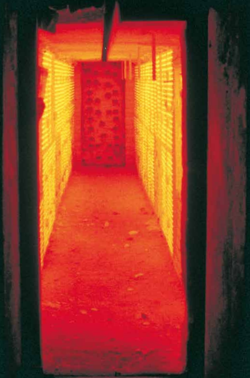
Fig. 19 Fibrothal modules in a suspended monorail furnace.
